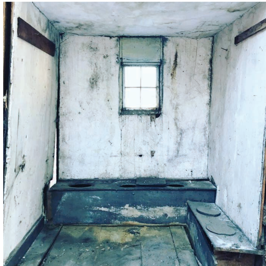
Recent construction work at the Harrington House revealed a five-holer privy that had been boarded over for decades.
