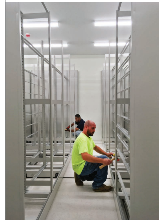
7 - Donnegan Systems, Inc. Installed our custom system over a week.
