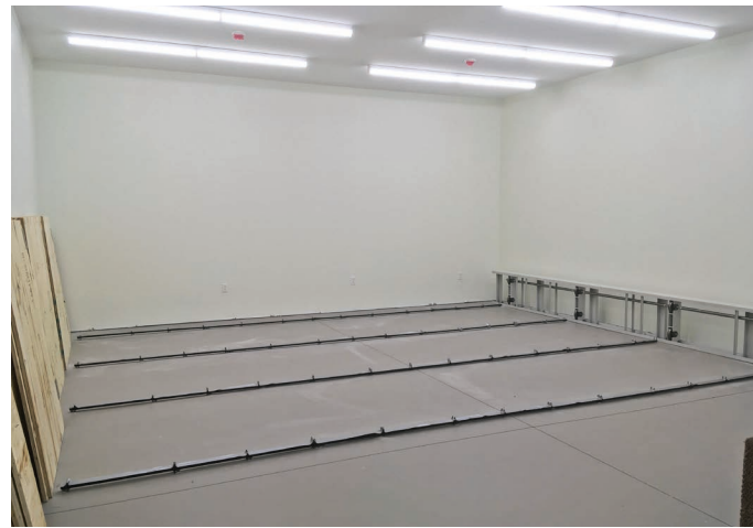
1 - The shelving rails for the mobile system.
