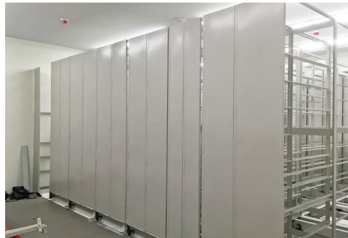
5 - The space starts to fill in with nearly 9-foot carriage fronts installed.
